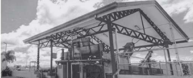
Baliwag Septage Treatment Plant WATER DISTRICT 120 m 3 /day
