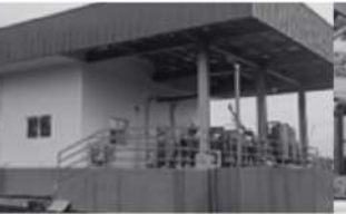
Metropolitan Naga WATER DISTRICT 60 m 3 /day
